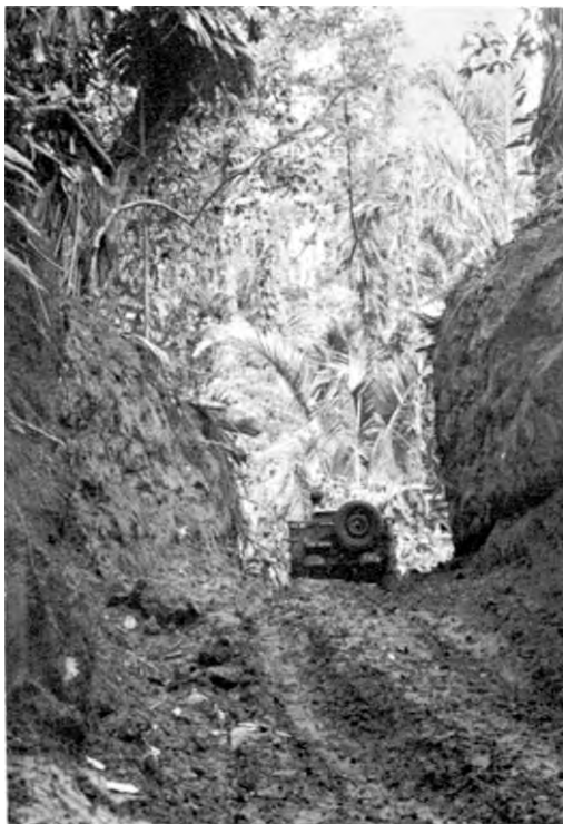
JEEP TRAIL FROM ZANANA, built through heavy jungle by 118th Engineer Battalion, 13 July 1943.
